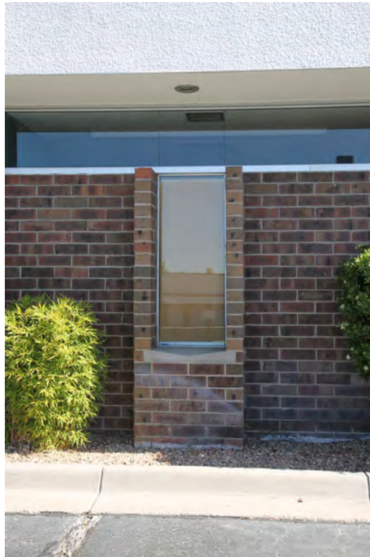
Granada Medical Plaza, north building, clerestory and window detail, photographer facing southwest
