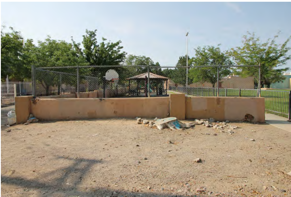
Photo 22. Adobe wall, playground, and bandstand north of Barelas Community Center, photographer facing south.
