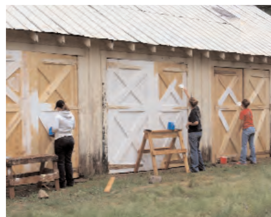
The YCC crew custom built and installed 11 wooden doors—each weighing over 100 pounds—into original openings on the north side of the barn and painted them. The barn is in Smokey Bear Ranger District.
